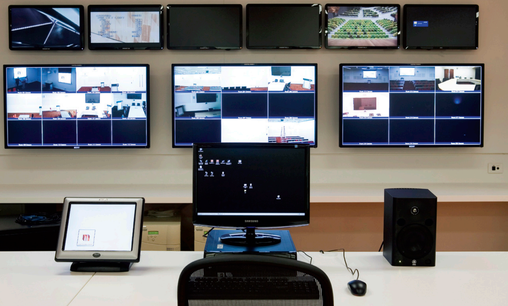
Master Control, showing monitor wall, master AMX Modero touch panel and control computer. The top row of monitors show (left to right) dedicated feeds from both cameras in the Grand Banquet room and all three Plenary cameras. The last monitor is a switchable preview of the in-house IPTV system. The three 47-inch LCD panels display the incoming meeting room camera feeds aggregated by the Avitech VCC-800c video command centres in each of the local control rooms. All video everywhere in the MCEC is full 1920 HD. The standard MCEC dual redundant uninterruptable power supplies can be seen nestled under the monitor wall.
