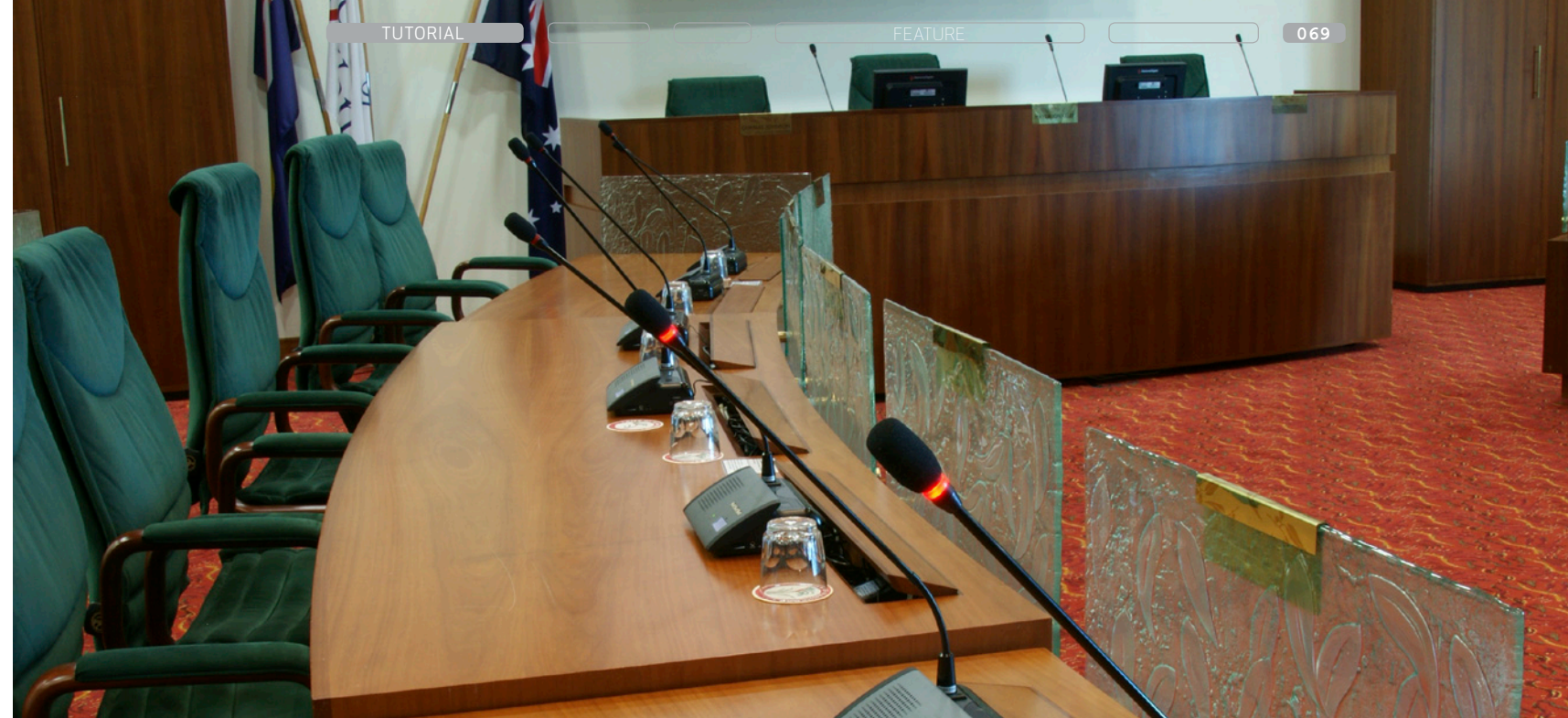
Multiple small low-level speakers and switched directional microphones minimise feedback and echo problems.
